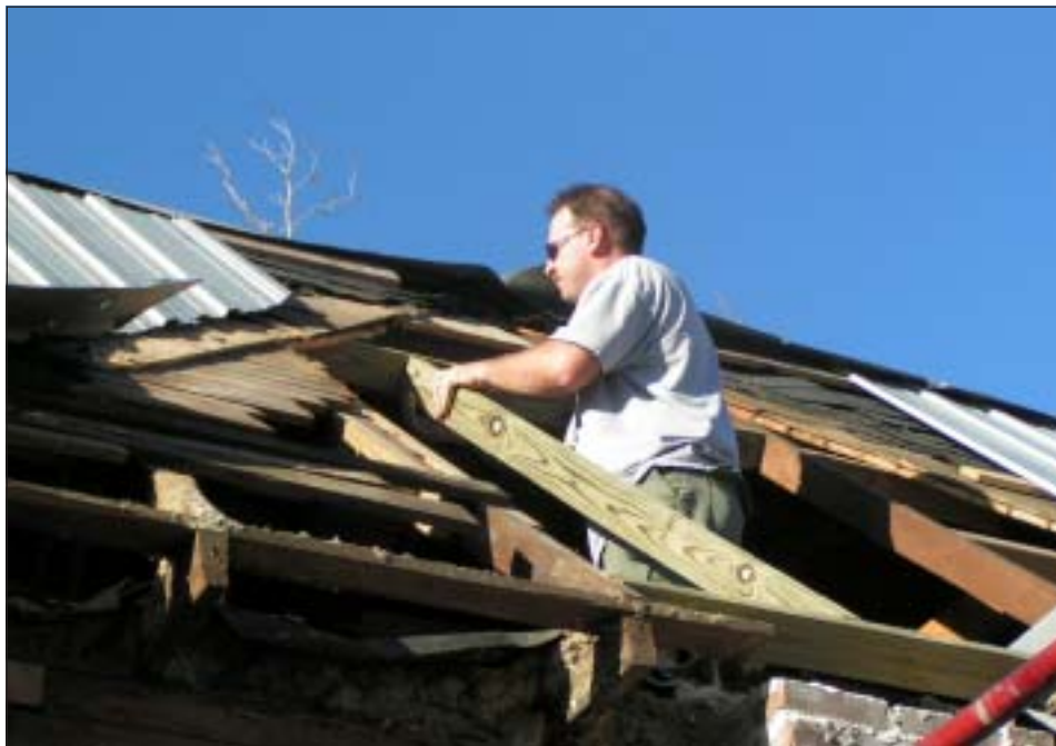
Master Sgt. Rick Little, 445th Airlift Wing Airlift Control Flight, repairs a roof on a home for a Hurricane Katrina victim in Mississippi. (Courtesy Photo)
