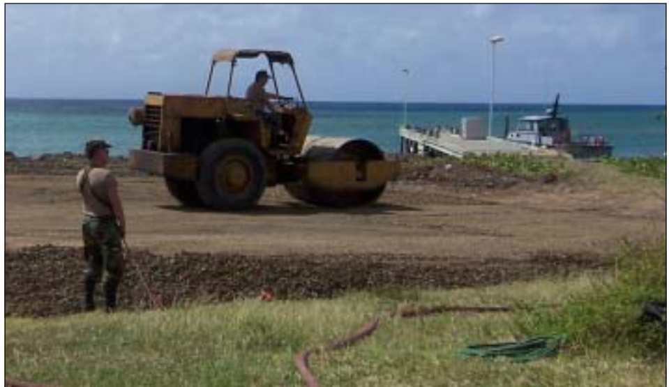
Tech. Sgt. Terry L. Lewis from the 445th CES Pavements and Heavy Equipment shop soaks the ground with water for the roller to compact. (Courtesy photo)
