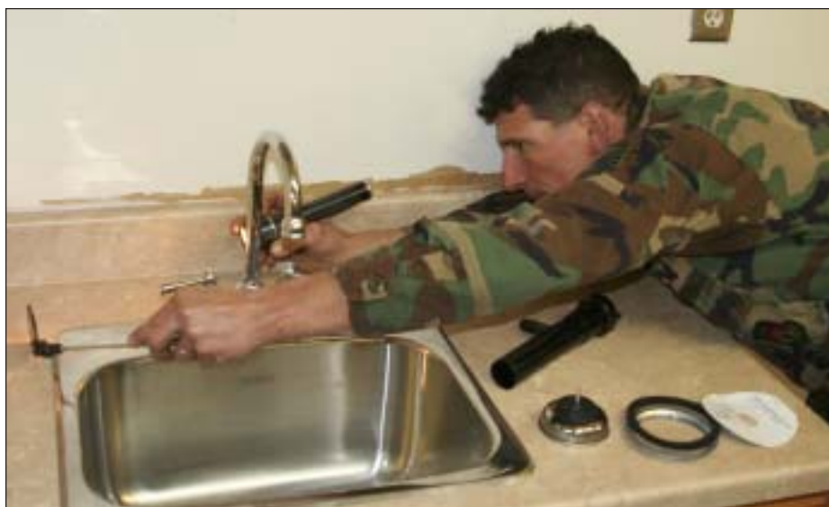
Master Sgt. Dennis Jones from the 445th Civil Engineer Squadron helps put in a new sink in the Airman Leadership Building. (photo by SrA Martin Moleski)
