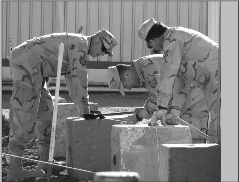
KIRKUK REGIONAL AIR BASE, Iraq - Left to right, Tech. Sgt. Clay Bucky, Master Sgt. Will Jobson and Tech. Sgt. John LeMaster, deployed from the 445th Civil Engineer Squadron, level concrete footings for a pod, which will house base Airmen. (U.S. Air Force courtesy photo)
