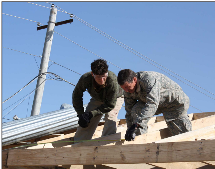
Tech. Sgt. Jonathan Lemaster, 445th Civil Engineer Squadron, works with a local Afghan craftsman as part of a new training program to recruit and certify local workers for construction projects on base. (Air Force photo/Master Sgt. Tracy Clare)
